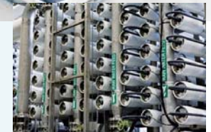
40,000 GPD(151.4 M 3 /Day) Leachate Treatment Plant Since 1997 , Oregon, USA
